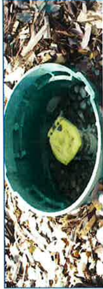
Quick coupler valves set 2-1/2" above finish grade in planting areas, placed centered within the valve box and anchored with an angle iron, 36" long.
