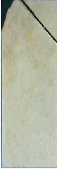
Medium broom finished concrete with clean, deep score joints spaced appropriately. No visible cracks or discoloration.
