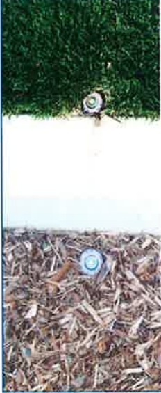
Irrigation heads at grade in planters and in turf areas.
