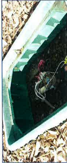
Valves placed centered in valve box, aligned square within the box, tagged and filled with drain rock.
