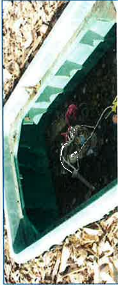
Valves placed centered in valve box, aligned square within the box, tagged and filled with drain rock.
