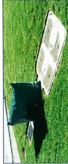
Backflow prevention device, meter and flow sensor are aligned.
