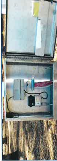
Irrigation enclosure contains equipment, neatly aligned. Manuals and irrigation station layouts are contained inside.
