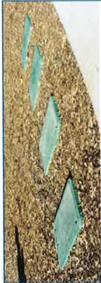
Valve boxes aligned and square with hardscape. Boxes are set at 2-1/2" above finish grade in planting areas and 1-1/2" above finish grade in turf areas.
