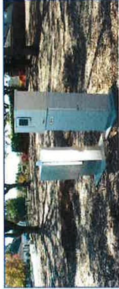
Electrical transformer and irrigation controller enclosure are aligned.
