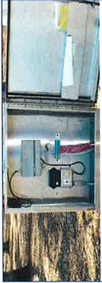
Irrigation enclosure contains equipment, neatly aligned. Manuals and irrigation station layouts are contained inside.
