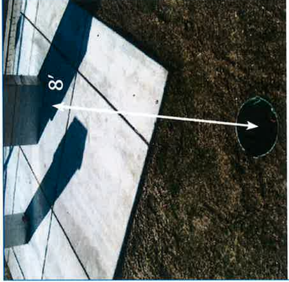
Ground rod 8' from control panel in irrigated areas.
