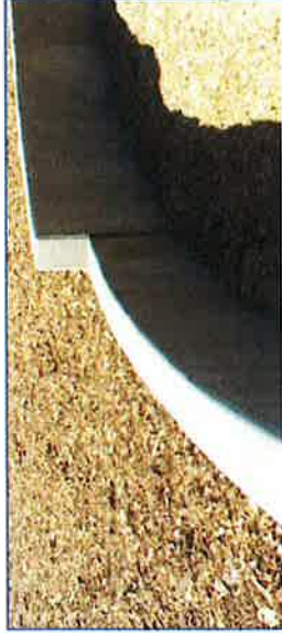
Vertical surfaces are consistent throughout. Vertical expansion joints are provided and are smooth with the finish surfaces. All edges have been eased at a consistent radius.
