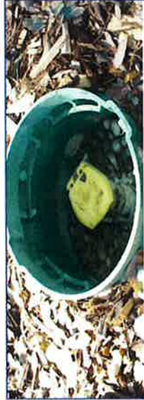
Quick coupler valves set 2-1/2" above finish grade in planting areas, placed centered within the valve box and anchored with an angle iron, 36" long.
